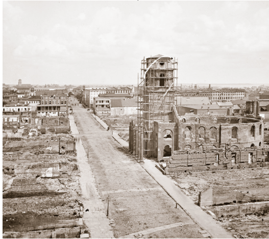
Above: Reconstruction meant a lot of rebuilding. This photograph of Charleston shows scaffolding on the shell of the Circular Congregational Church on Meeting Street.
